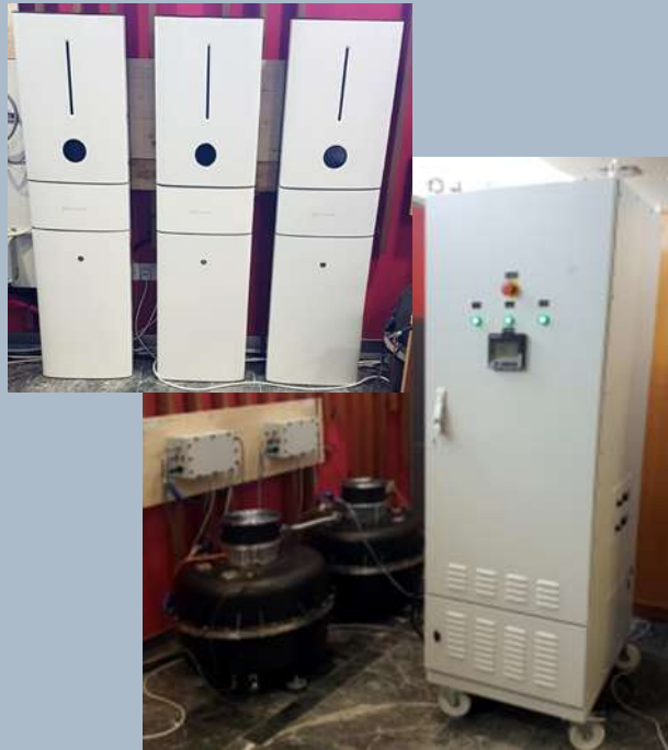
Pilot II: Battery & Flywheel storage system at KIOS CoE
