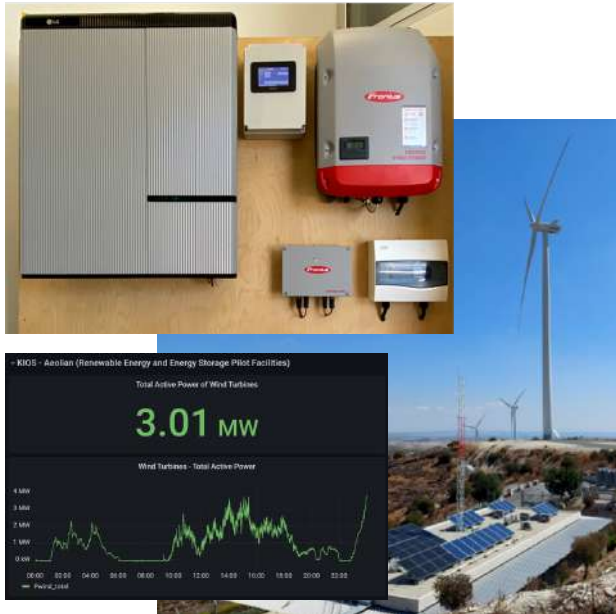
Pilot I: Battery storage system at Aeolian Dynamics
