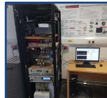
Prototype Storage Inverter
